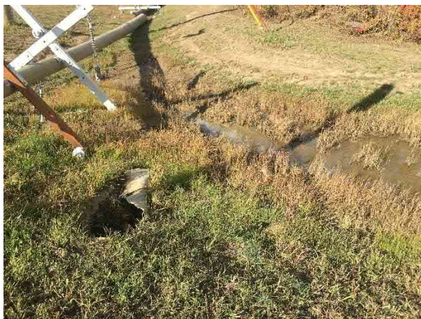
Figure 11 – Smashed culvert in NE corner
