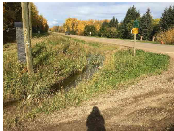
Figure 12 – Ponding in NW corner
